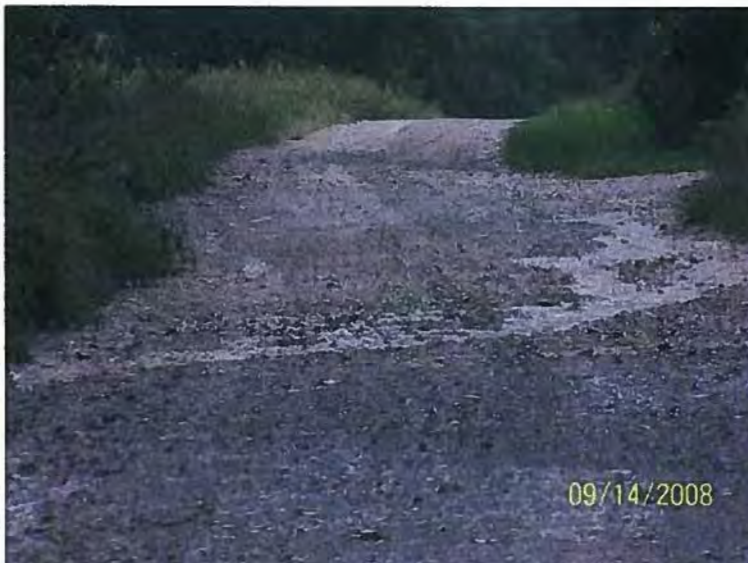
WATER RUNNING OUT OF THE HILLTOP CONFINEMENT DRIVEWAY NEXT TO CULVERT RUNNING DOWN THE ROAD TO SUGARCREEK IN ABOVE PICTURE
