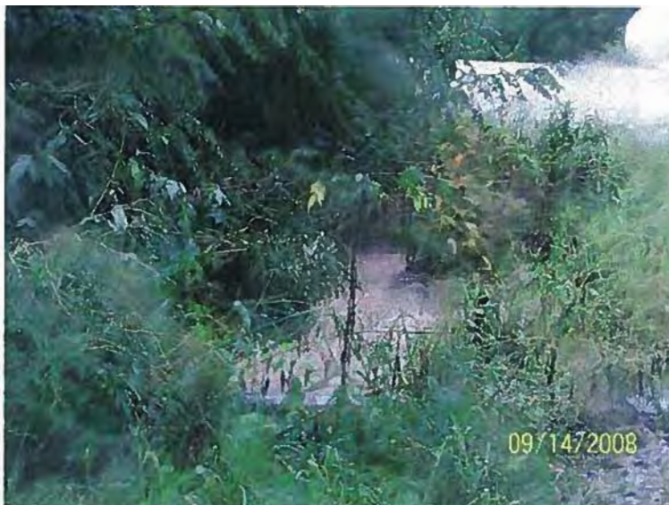
CULVERT NEXT TO THE HILLTOP ENTRANCE RAIN RUN OFF DRAINING INTO DITCH
